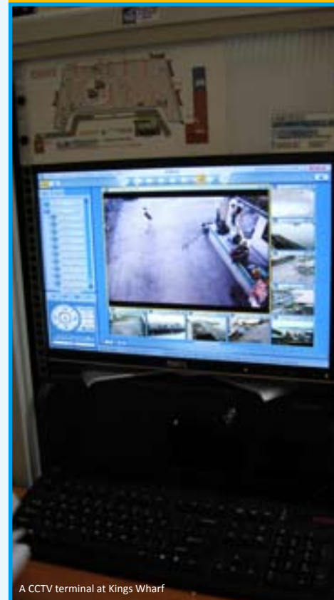
A CCTV terminal at Kings Wharf
